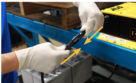
Figure 4: Reconnect AC power to the charger
